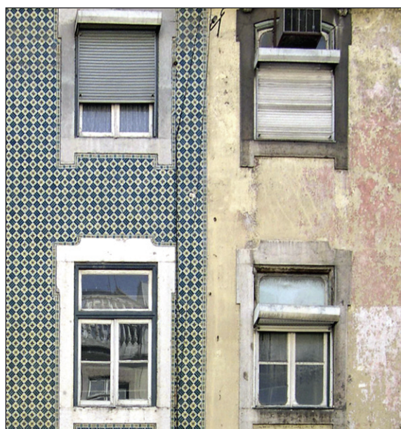
Figure 19 Glazed tiles have a superior durability comparing with traditional plaster with paint coating
