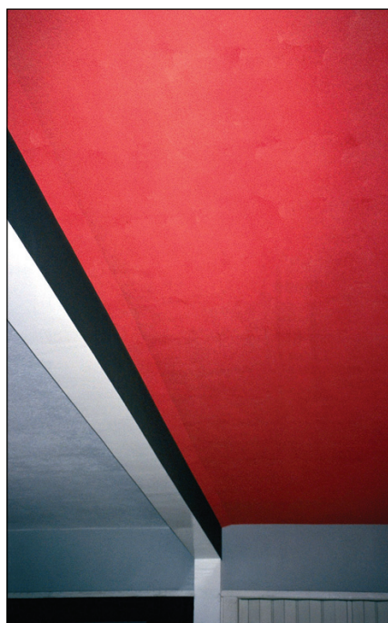
Figure 3 The Bauhaus school in Dessau (Gropius, 1925–26) is full of contrasts in colour, gloss and surface texture (ceiling in canteen building)
