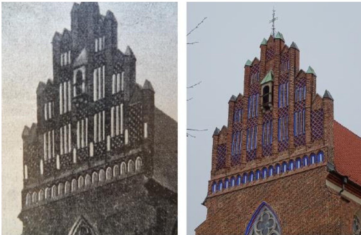
Figure 5: The Corpus Christi church, Wrocław. The medieval gable was painted in the 1920s (left). By Schlesischer Malerbund, 1928, vol. 11, 367-369. The detected colour scheme was restored a few years ago (right). Photo by the author, 2014.
