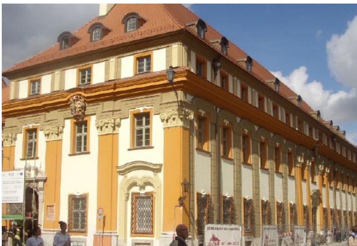
Figure 9: The former orphanage at 4 ulica Katedralna, Wrocław was restored to one of two colour schemes suggested by a conservator who made an on-site examination (Photo by the author, 2012).
