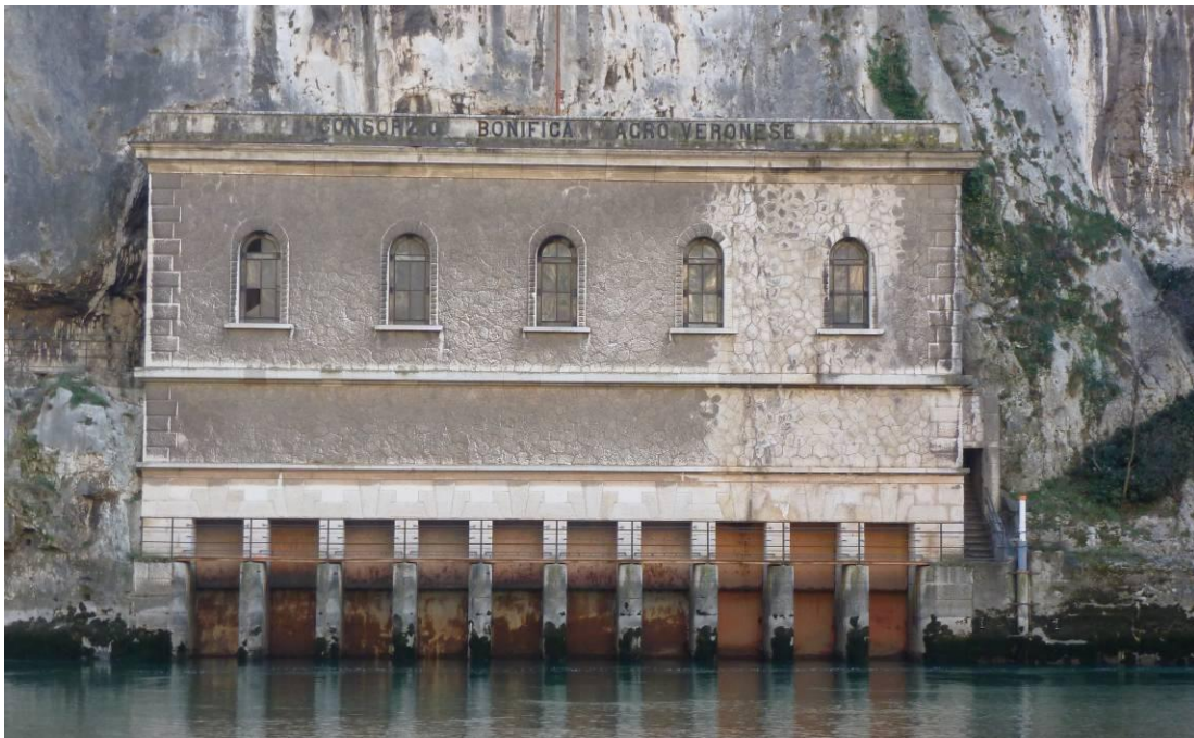
Fig.6 – Chiusa di Ceraino, Rivoli Veronese, VR. Cladding system in pinkish stone, with different textures, iron frames with glass panels such as "cathedral" with blue inserts. The floodgates are made of metal rusty reddish in color. The original floodgates were made of wood. (foto © K.Gasparini)
