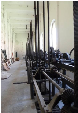
Fig.7 – Chiusa di Ceraino. Focus on the plants originating in iron casting: in the white color of the wall paint the emerging the color of black paint and rusty metal (foto © K.Gasparini)
