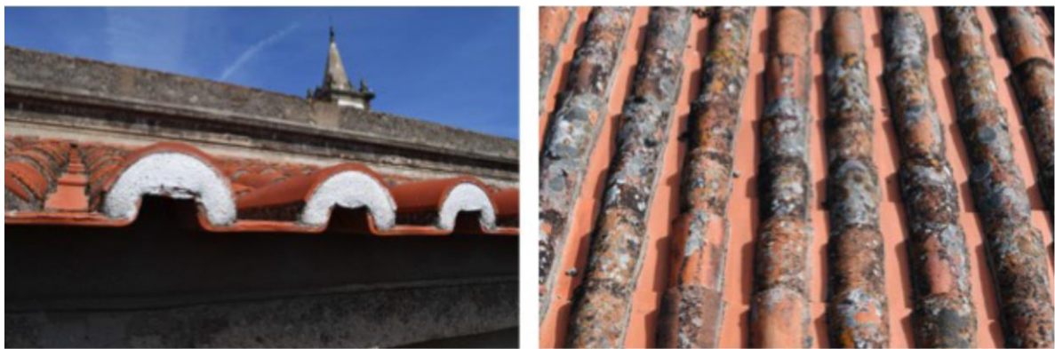
Figure 5: Cathedral of Portalegre : existing roof in ceramic roof tiles called Roman tiles. Photos by RBD.APP, 2016.
