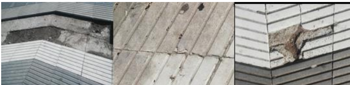
Figure 2: Missing tiles (left), dust accumulation (center), broken tiles (right). © 2003 Sebastián Marquez. All rights reserved.
