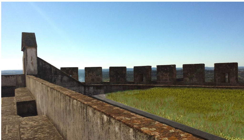
Figure 1: Portalegre Cathedral: Terrace View to the Green Roof of the Permanent Exhibition Room in the southwest courtyard. Rehabilitation made by RBD.APP, 2016.
